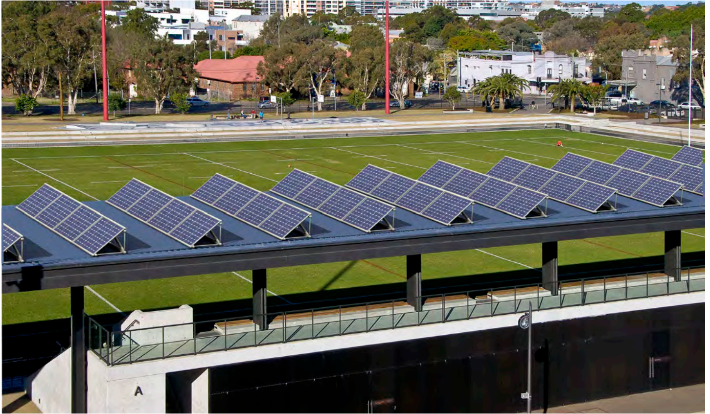
Solar panels installed on the roof of Redfern Park
